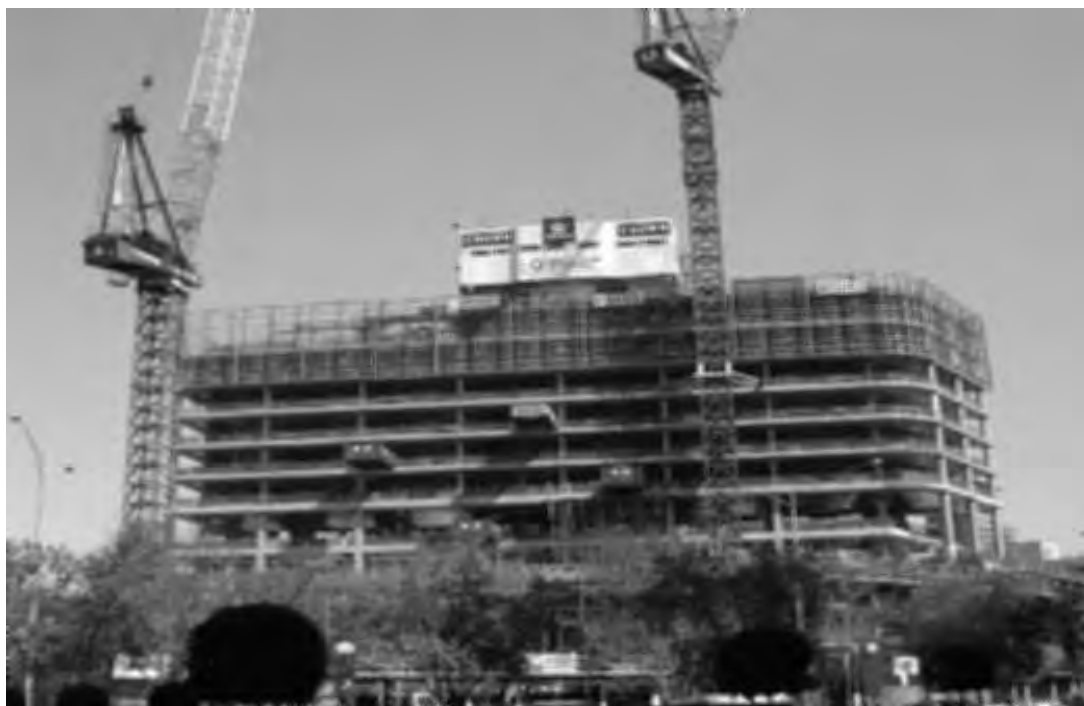
Progress of the construction of a second hotel tower at the casino complex.
